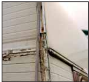
Check for failed mastic
