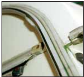
Rusting screws may mean water leaks
